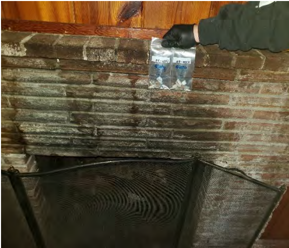
Photo #13: Samples 11720-76 & 77: Red external fireplace brick and gray internal fireplace brick on ACM mortar. (4% Chrysotile) Location: Building 6 Living Room
