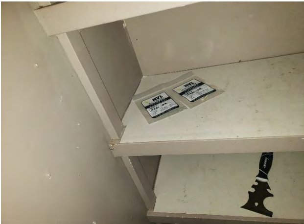
Photo #1: Samples 11720-05/05QA & 06: Beige joint compound (on GWB.) (3% Chrysotile) Location: Building 8 Kitchen
