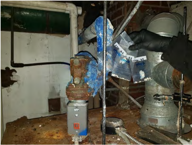
Photo #9: Samples 11720-62,63 & 64: Blue and white mudded elbows (on 4" OD metal boiler piping.) (12% Chrysotile, 5% Amosite) Location: Building 7 Garage Area
