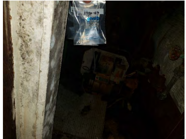
Photo #10: Samples 11720-67, 68 & 69: TSI lining (on boiler interior.) (85% Chrysotile) Location: Building 7 Garage Area
