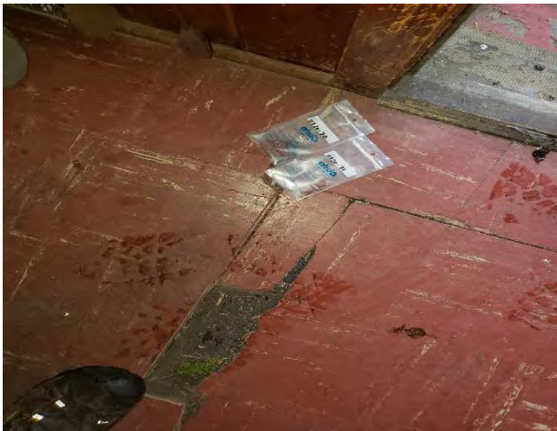
Photo #11: Samples 11720-70,71/71QA: 9"x9" Red VFT on black mastic (on wood.) (5% Chrysotile, <1% Chrysotile) Location: Building 6 Living Room
