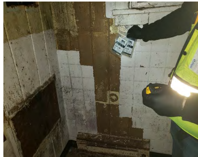
Photo #8: Samples 11720-50 & 51: 4"x4" White ceramic tile on gray grout on brown mastic (on wood paneling.) (4% Chrysotile) Location: Building 9 Bathroom
