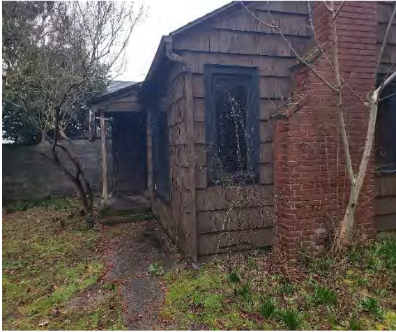
Photo #17: Assumed ACM red and gray fireplace brick with mortar. Location: Throughout Building 2-4
