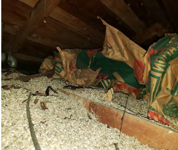
Photo #15: Assumed ACM vermiculite insulation. Location: Building 6 Attic Space South
