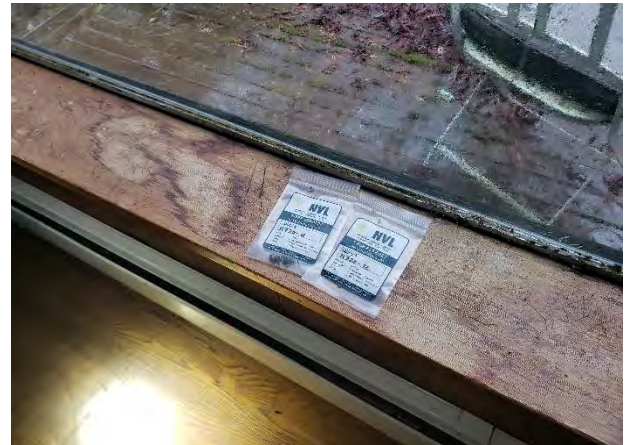
Photo #2: Samples 11720-11/11QA & 12: White interior window glazing (on 9'x11' metal frame window.) (4% Chrysotile) Location: Building 8 Living Room Interior
