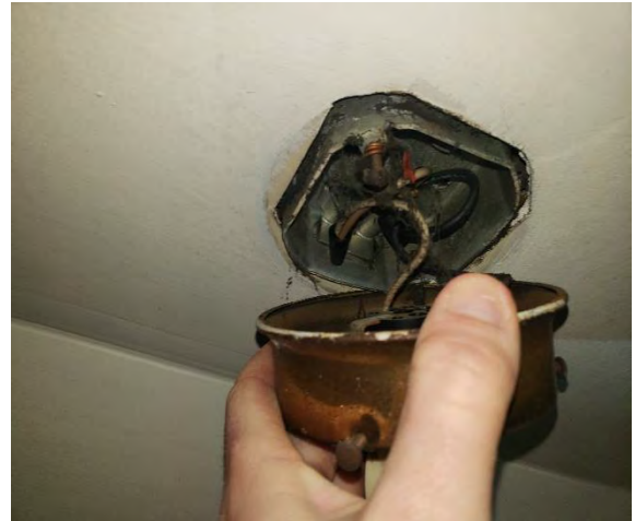
Photo #16: Assumed ACM cloth insulated electrical wiring. Location: Throughout Buildings 2-9
