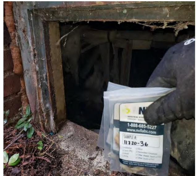
Photo #4: Sample 11720-36 through 38 & 60/60QA & 61: TSI (on 3" OD metal hot water piping.) (44% Chrysotile) Location: Building 8 Crawl Space and East Garage Building
