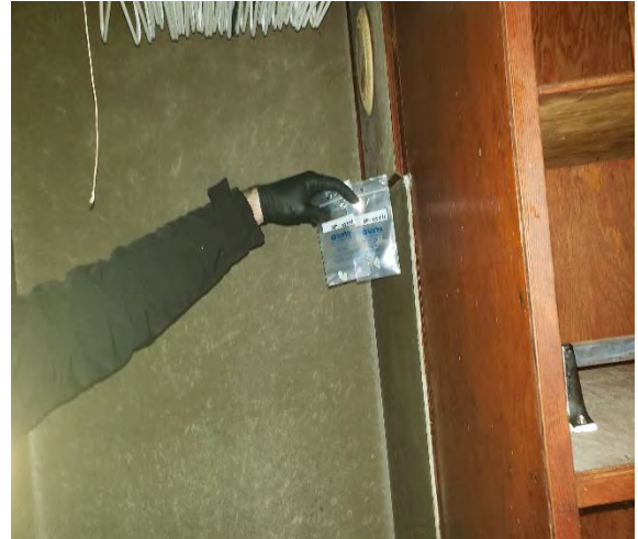
Photo #14: Samples 11720-91 & 92: Dark gray cement board paneling (on wood.) (31% Chrysotile) Location: Building 5 Bathroom Exterior
