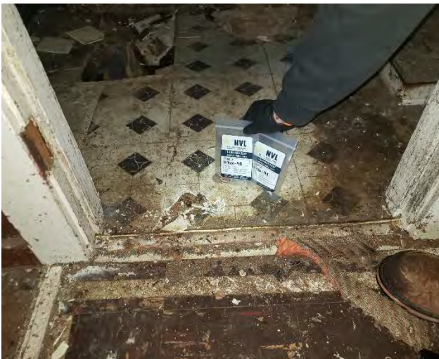
Photo #7: Samples 11720-48 & 49: 12"x12" White and black VFT on brown mastic (on wood) (46% Chrysotile) Location: Building 9 Bathroom
